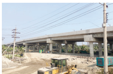
Construction Supervision of 2 lanes Flyover as extension part of the existing flyover at Mohonpur rail crossing under the project Integrated urban infrastructure development in Rajshahi city
